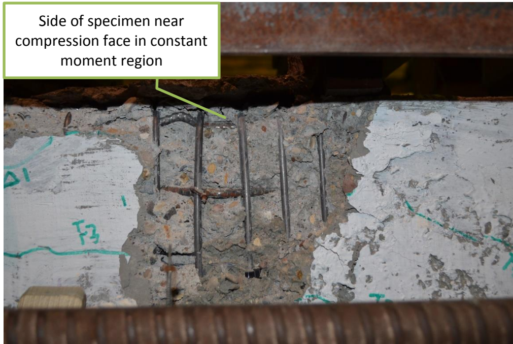
Figure 5-66: Specimen H2S1-M Longitudinal Reinforcement Buckling after Failure
