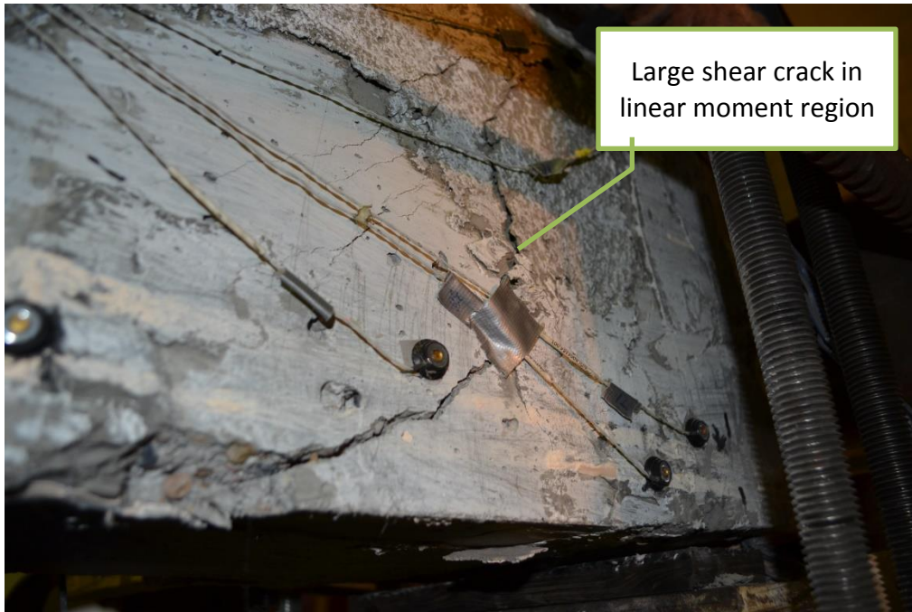
Figure 5-69: Large Shear Crack in the Linear Moment Region on LED Side of Specimen H2S2-C after Failure
