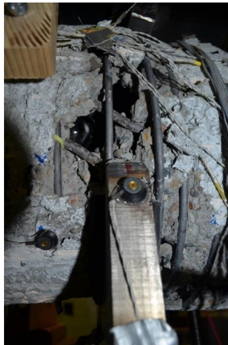
Figure 5-19: Specimen H1C3-C Close-Up of Local Failure on LED Side after Clearing Damaged Concrete
