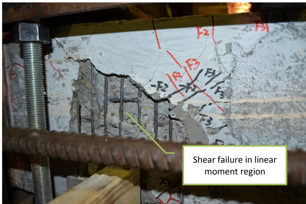
Figure 5-68: Specimen H2S2-C Shear Failure in the Linear Moment Region
