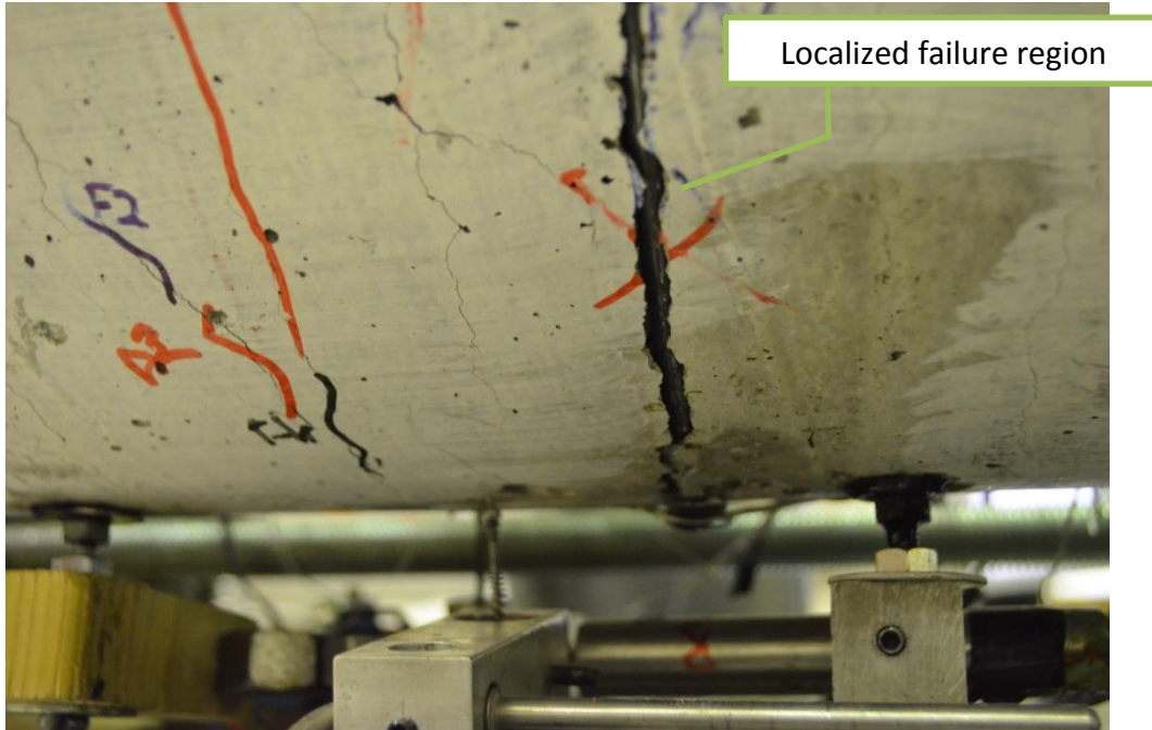
Figure 5-5: Large Flexural Crack in Specimen SC1-M at End of Test
